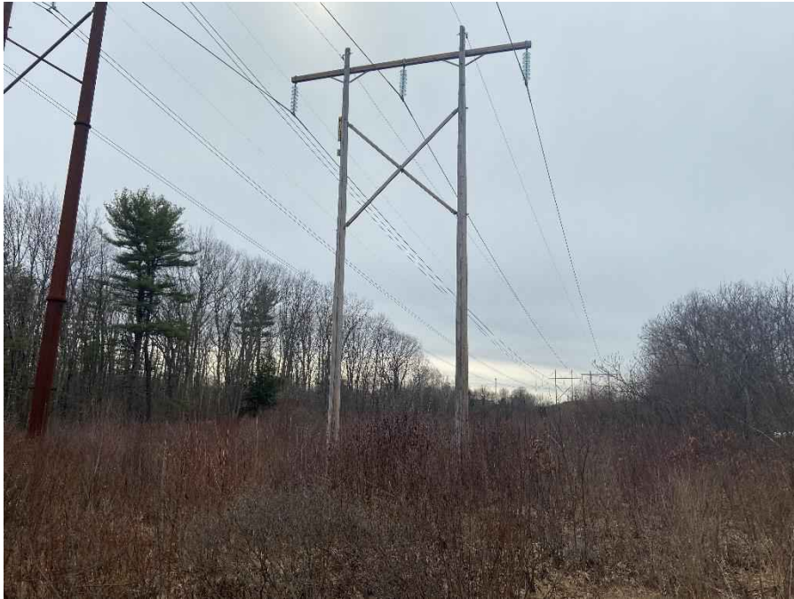
Photograph No. 3: Looking northerly from Evans Road at M183 Structure 4 to be replaced.
